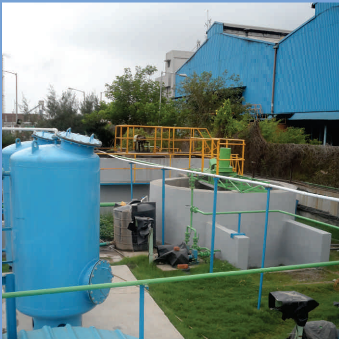
Sewage Treatment Plant - Moraiya Unit
